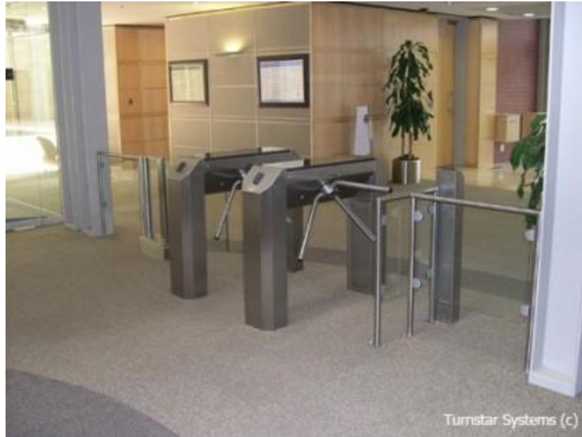
Figure i: Typical installation with barriers and screen
